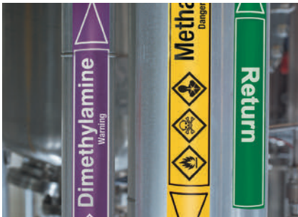
Pipe & valve marking
