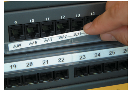
Punch block & patch panel labels
